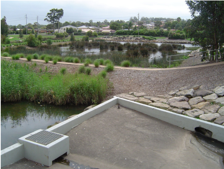
Figure 2.6.8. Constructed wetlands may contain many different components, each bringing with them a different suite of mosquito risk factors. All components of a wetland, as well as surrounding habitats, should be taken into account when reviewing design plans and mosquito monitoring programs. (Photo: Cameron Webb, Medical Entomology, Pathology West – ICPMR Westmead.)
